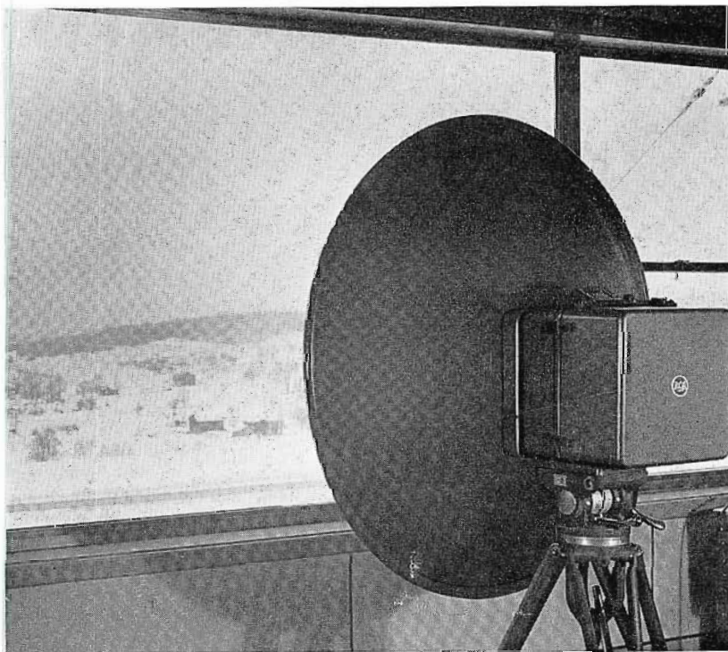
FIG. 9. Spare microwave receiver is mounted in the main transmitter room—conventional tripod allows movement for remote pickups.
